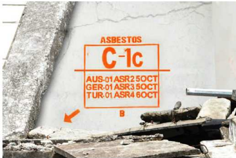
Figure 23: Turkey 01 having completed ASR 4 Full SAR on the worksite, have determined no further work is required on this worksite.
